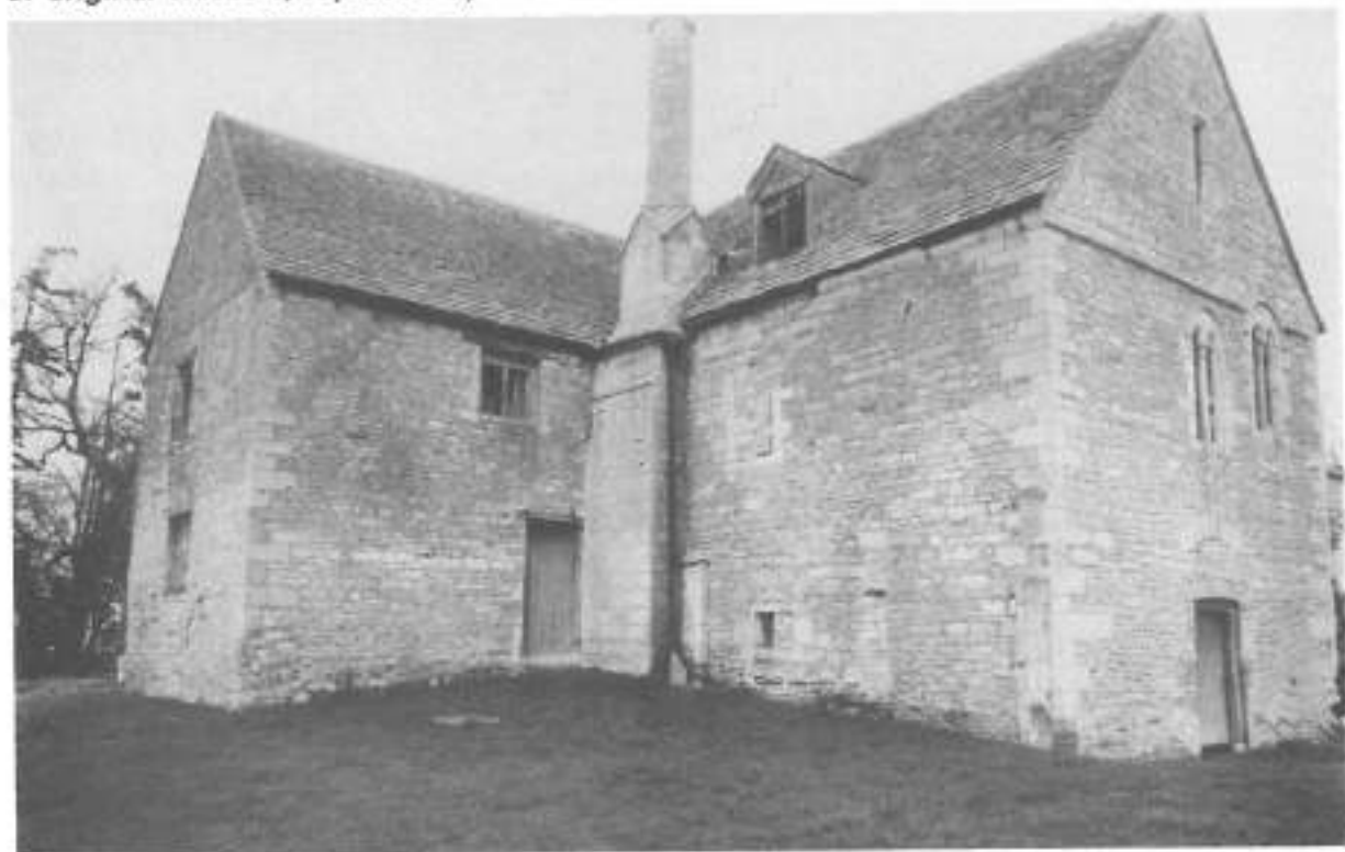
South west view showing chimney, blocked windows in west wall, and later westward extension.
