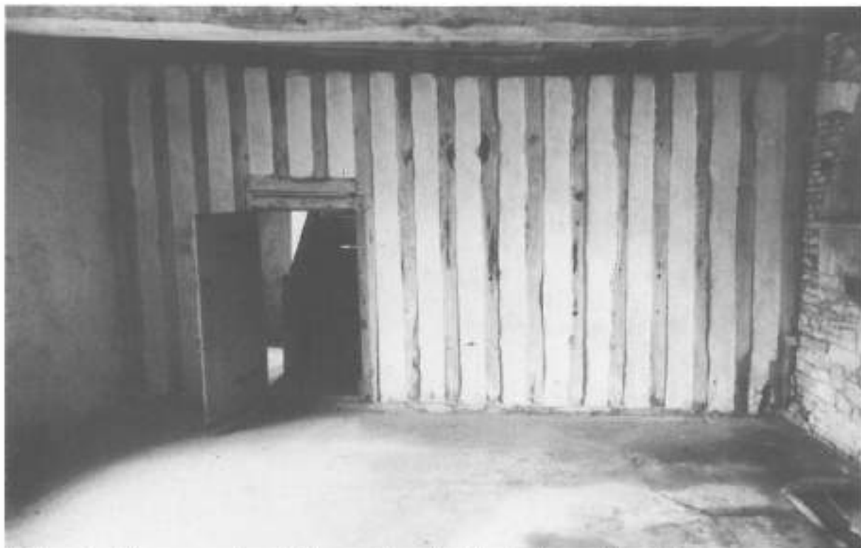
Timber studding screening off the south end of the hall, possibly 15th century.
